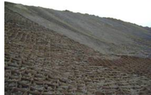
Barren slope after drainage works
